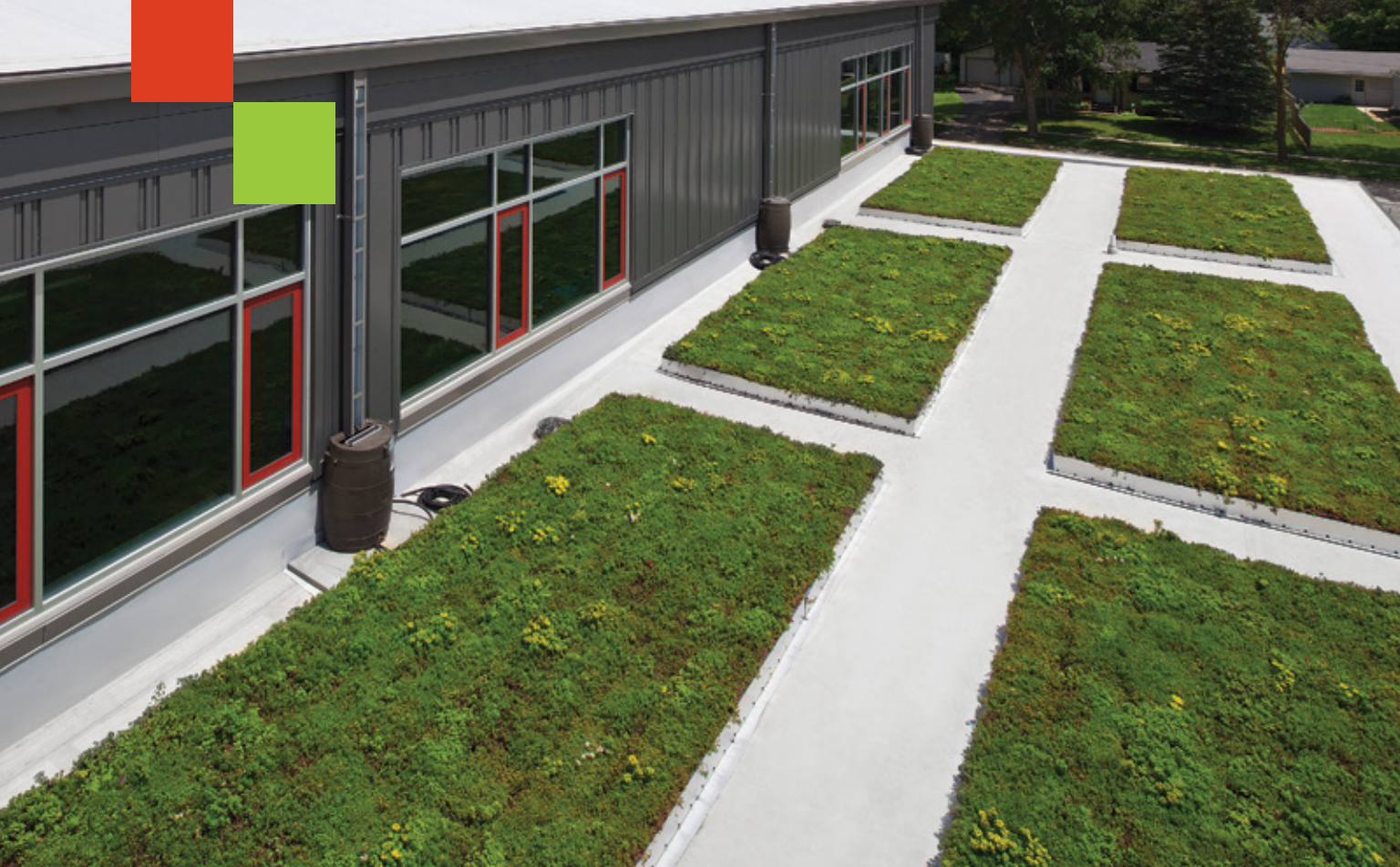
Windows overlook a green roof at Lake Mills Elementary School, allowing teachers to use the roof as a teaching tool for their students.
