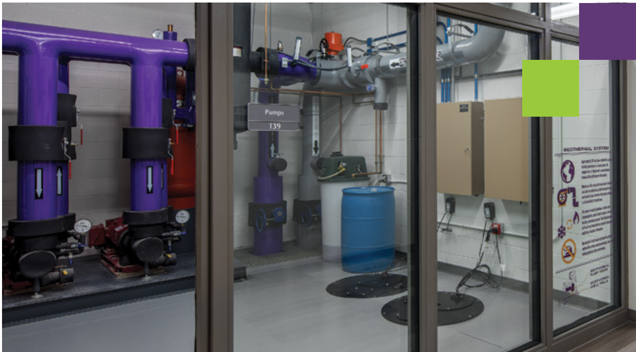
Waunakee Intermediate School students can peer into the geothermal pump room and learn more about how the system works from the nearby window graphic.
